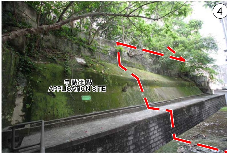
從新村街50號西面方向望向申請地點的景觀 WESTERN VIEW OF THE APPLICATION SITE FROM 50 SUN CHUN STREET
