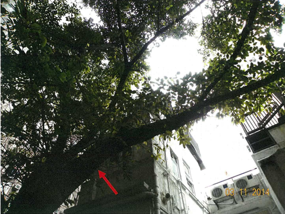
T1's large limb (approx. 400 mm diameter) conflicting with future 3/F building wall – 1
