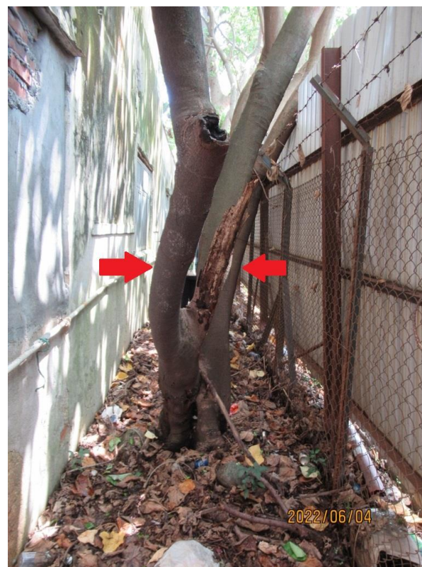
T9 Trunk Condition - FELL
