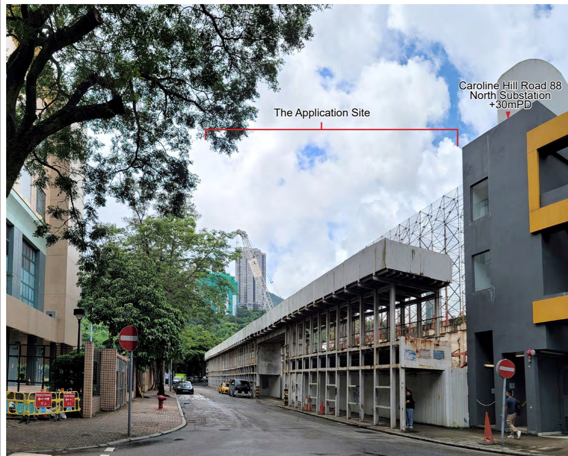
Existing View View southeast from the junction of Caroline Hill Road & Cotton Path
