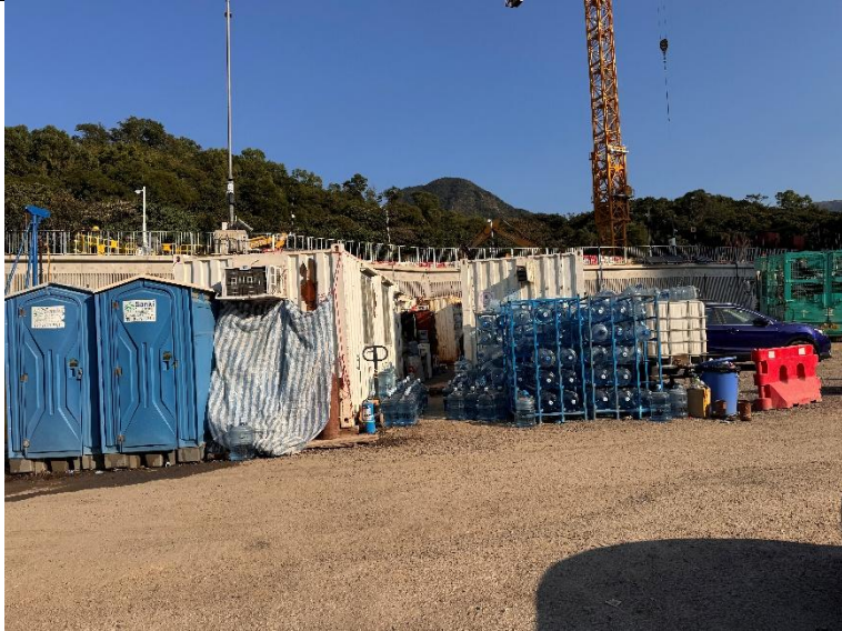
Photo 9: Containers are observed but there is no direct contact between the container and the ground. Temporary toilets and water bottles are observed too. The area is covered in sand in good condition. No oil stains and smells are observed.
