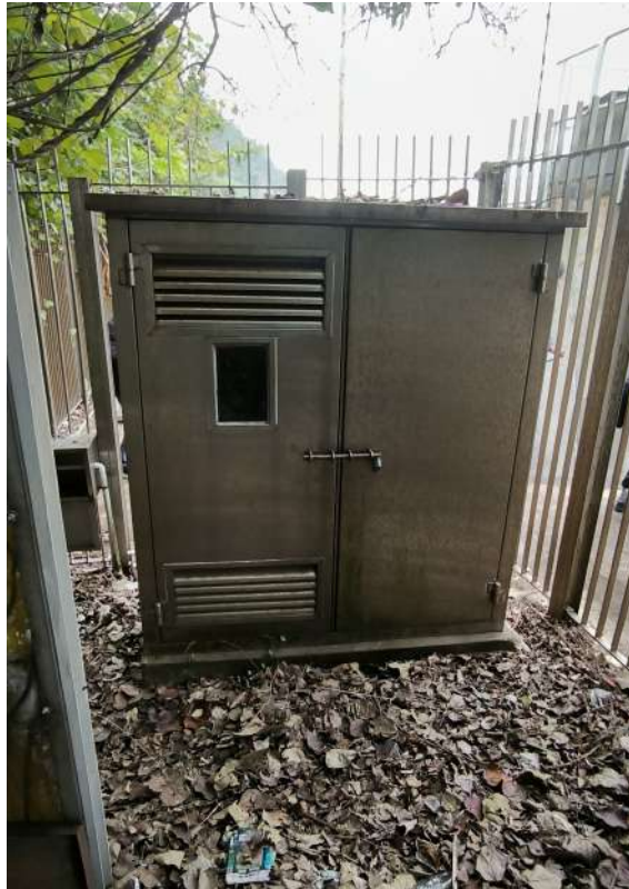
Figure 15: Power box close to the Facility gate.
