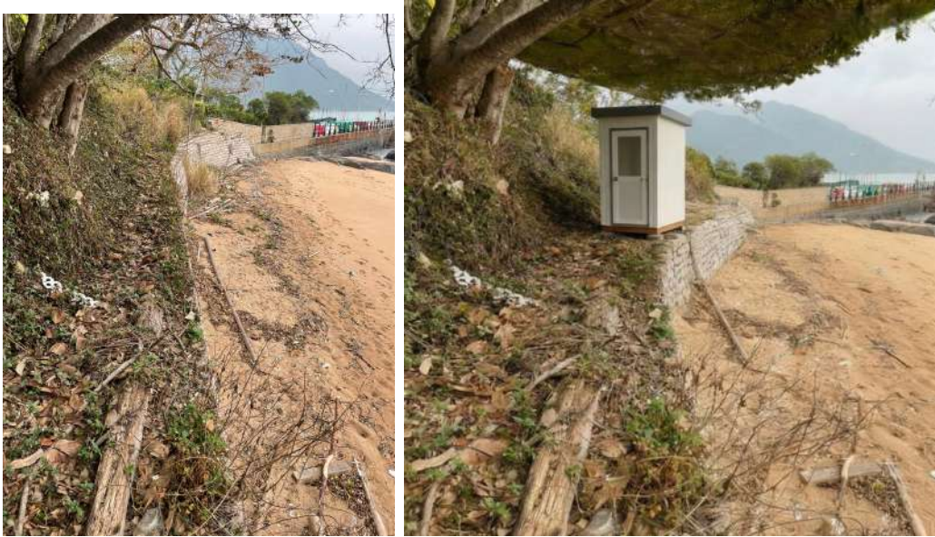
Figure 24: Left panel: Current state of the retaining wall and surrounding landscape. Right panel: AI-generated rendering illustrating the placement of the server cabin above the wall, designed to preserve existing canopy trees.
