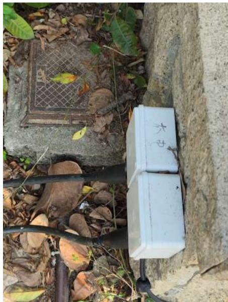
Figure 25: Existing supply points attached to the wall at the boundary of the beach.
