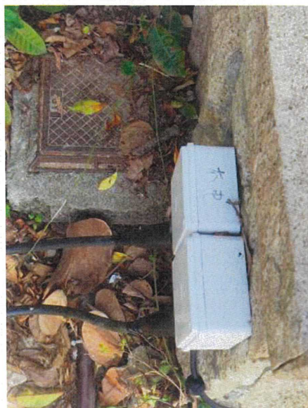
Figure 25: Existing supply points attached to the wall at the boundary of the beach.
