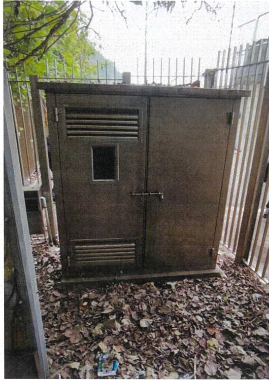
Figure 15: Power box close to the Facility gate.
