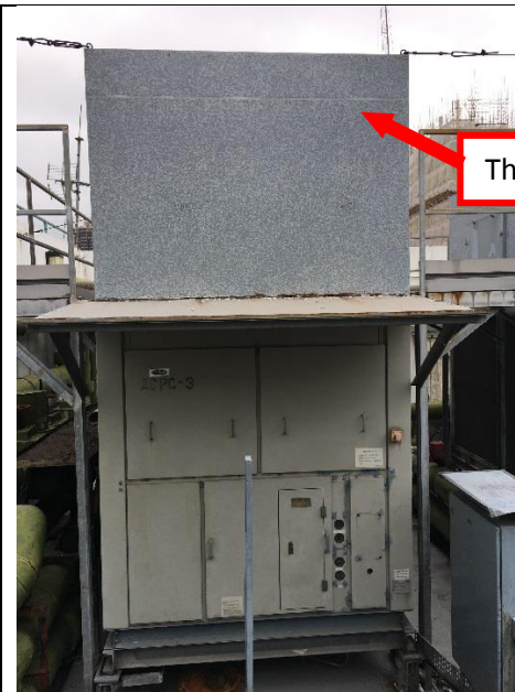
Side view, the brand of chiller is Carrier.
