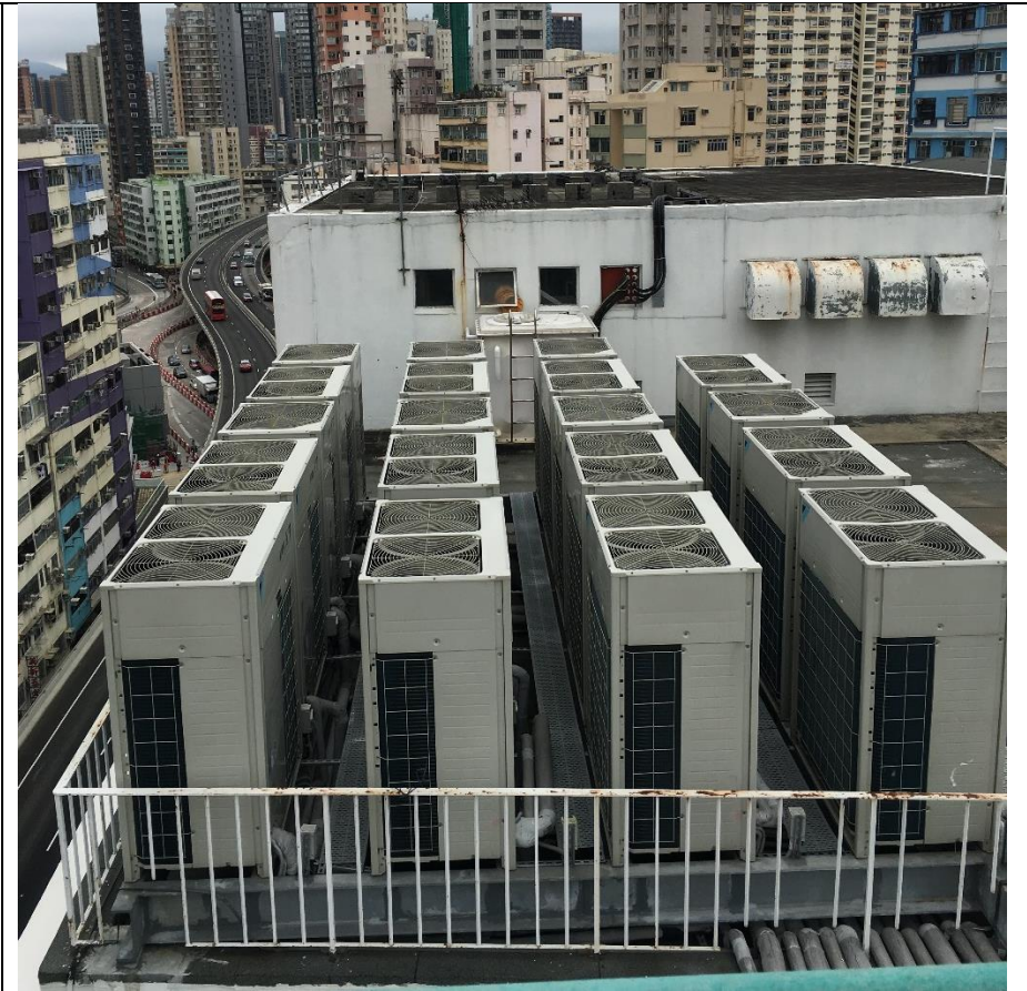
There are in total 19 nos. of VRVs on the roof of BMW house. 12 nos. of VRVs have double top fan, 7 nos. of them have single top fan. Their location is indicated in Figure 4.2 .
