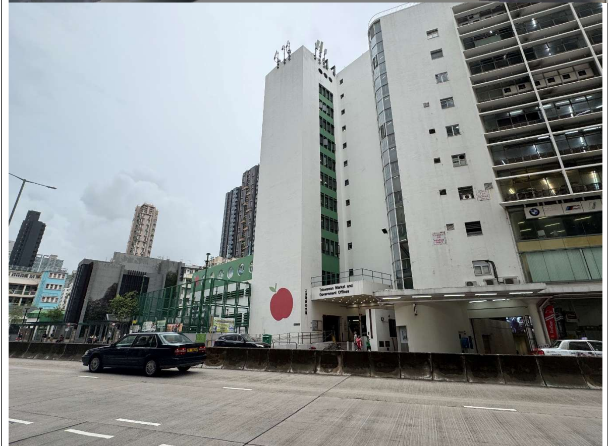
C01 to C05 To Kwa Wan Complex and Government Offices – Chillers and VRVs No nighttime operation (23:00 – 07:00) SWL reference from EA report of CBS:2-KC
