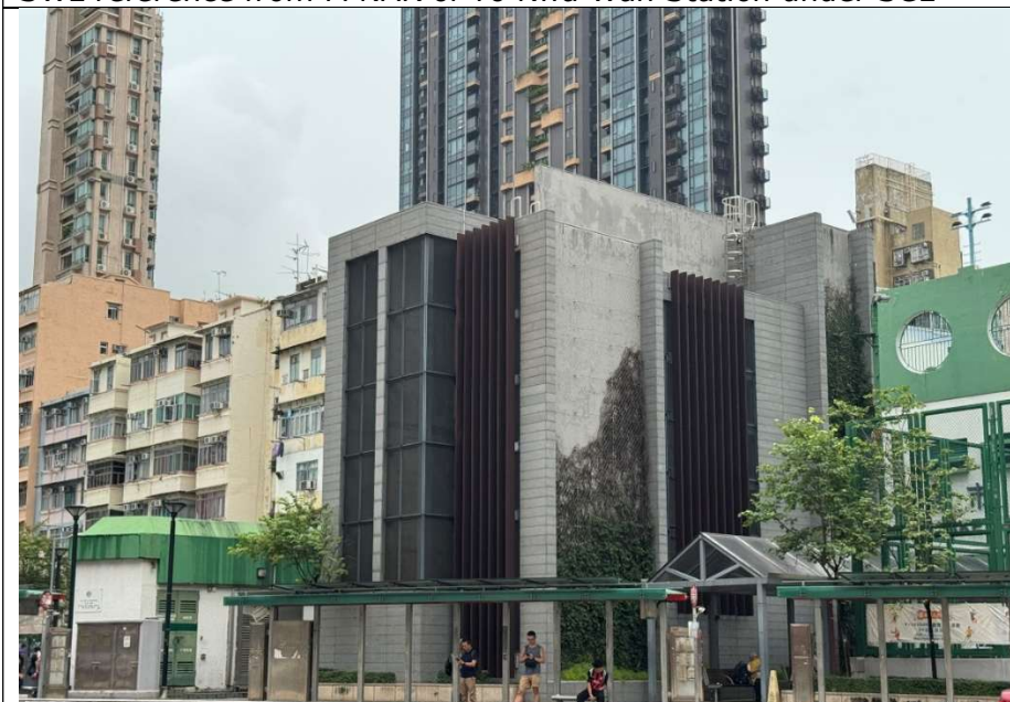
F01 to F14 Ventilation Shaft (next to To Kwa Wan Market) – Ventilation Louvre Operation follow MTR operation hour (Both daytime & evening time and night-time operation) SWL reference from FPNAR of To Kwa Wan Station under SCL
