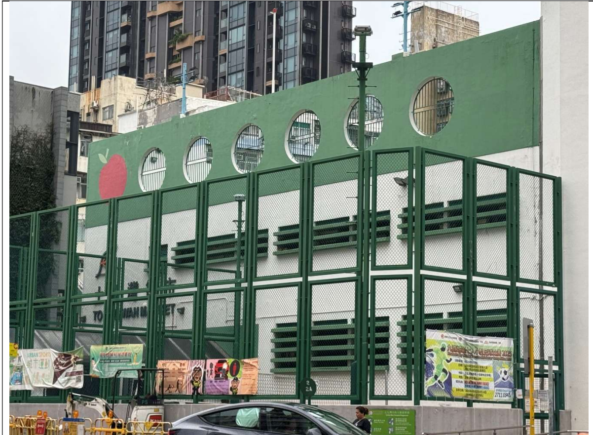
A01 to A07 To Kwa Wan Market – Chillers and VRVs No nighttime operation (23:00 – 07:00) SWL reference from reference EA report of CBS:2-KC
