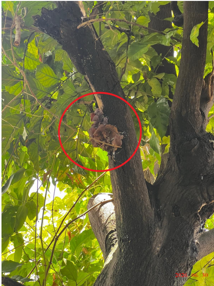
9. Branches condition_fungal fruiting bodies_closeup
