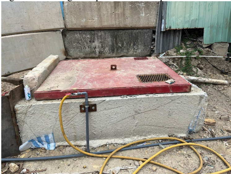
Figure 1. Existing catchpit with sand trap #1
