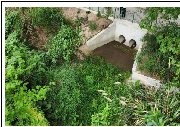
Photo No. 5 – Existing stormwater inlet under the elevated Heung Yuen Wai Highway from which the flow will pass through twin 900mm diameter drains and go to the west
