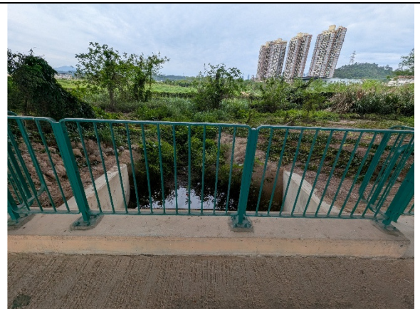
Photo No. 6 – View toward the downstream of the existing stormwater inlet under the elevated Heung Yuen Wai Highway
