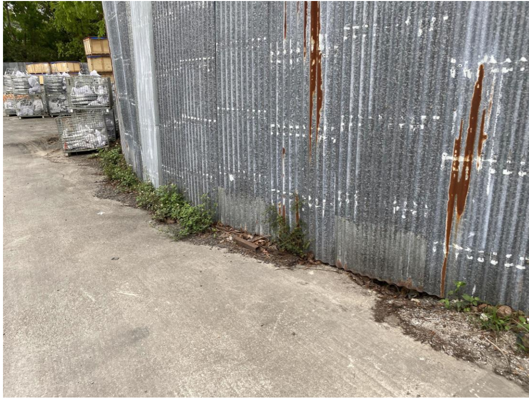
Photo 1: Hoarding without concrete footing
