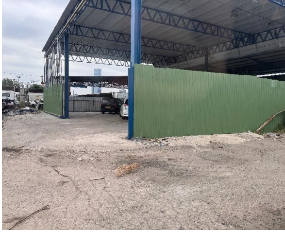
Photo 7: The area is used for temporary car parking. No car repairing activities are observed. The ground is paved with concrete with some cracks observed.
