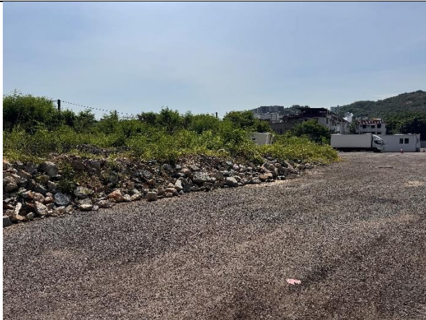
Photo 5: The ground is paved with concrete in good condition. Some tyre marks are observed.
