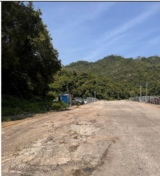
Photo 17: The ground is paved with concrete with some cracks are observed
