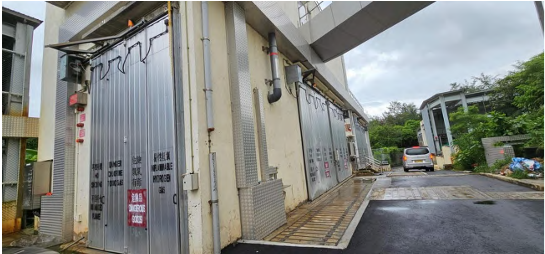
FIGURE 10 Site Photo 5 - Existing On-site Chlorine Generation
