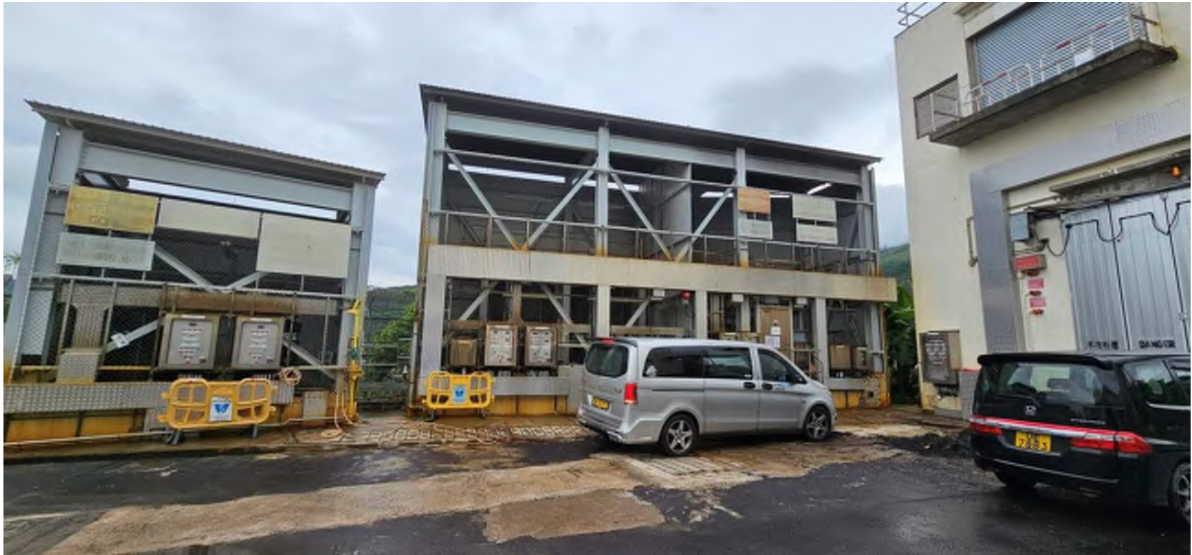
Site Photo 6 - Existing On-site Chlorine Generation
