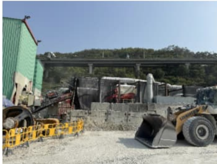
PHOTO 3251: CRUSHING AND SCREENING FACILITIES (DATE TAKEN: 8 APRIL 2025)
