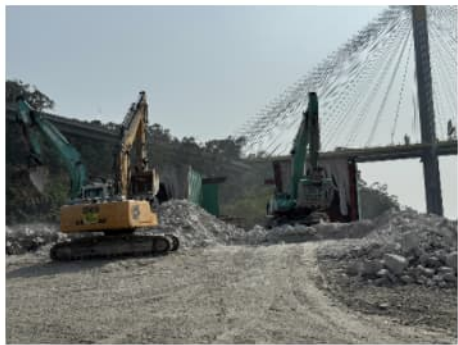
PHOTO 3220: UNLOADING PLATFORM AND HOPPER (DATE TAKEN: 8 APRIL 2025)
