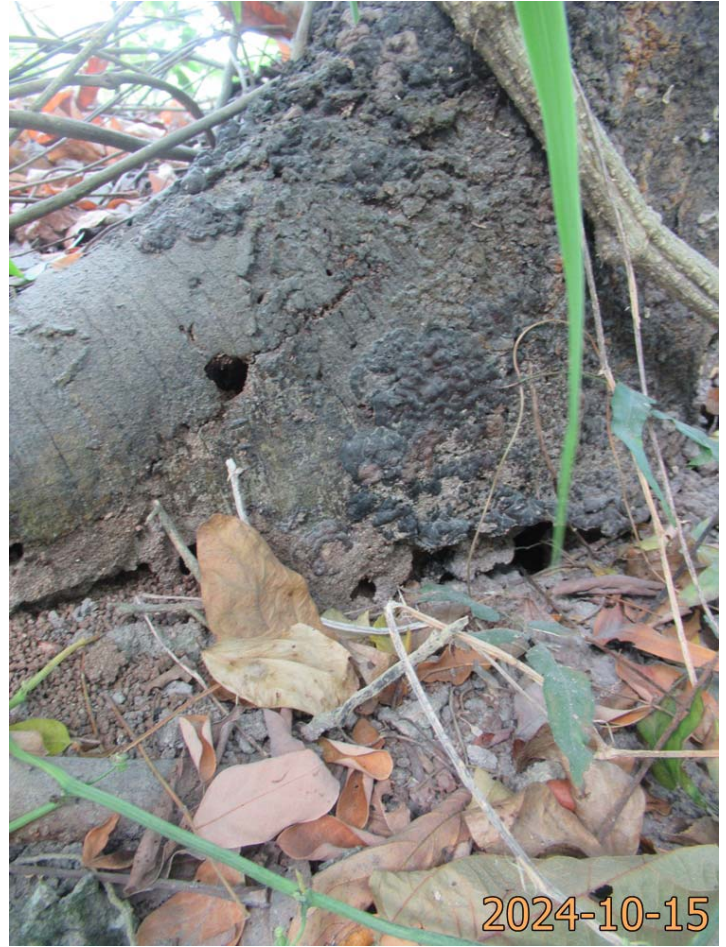
T15 Trace of termite
