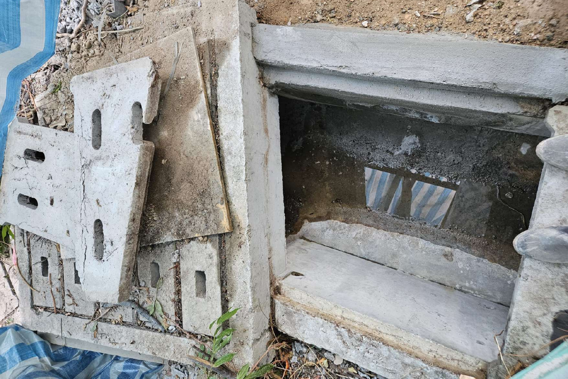
Photo 1 : 750mm Surface Channel
