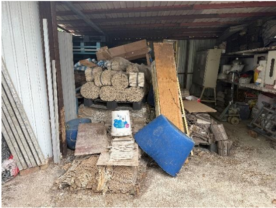
Photo 13: Temporary storage of construction materials including used timber, empty containers, tarpaulin sheets, tiles within the temporary structure
