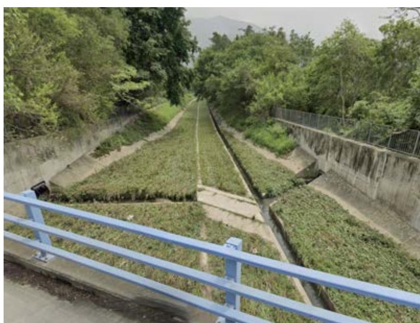
Final Discharge Point
