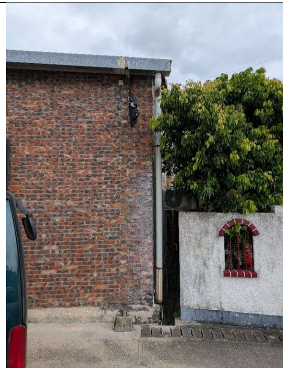
Plate 8 – Existing 225mm channel running along the northern boundary of the Application Site with existing gutter at the roof edge discharging into the existing channel.
