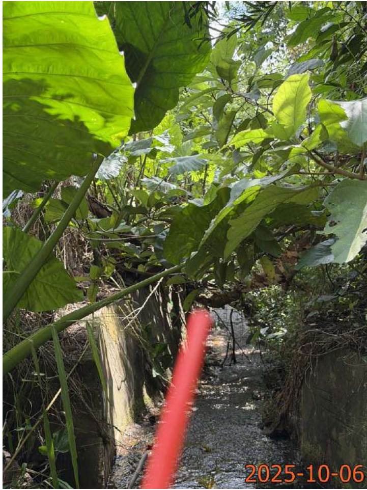
T10 (Overview) (Collapsed)
