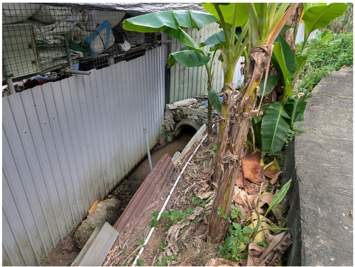
Photo No. 12 – Close up view at an existing drain at the existing watercourse
