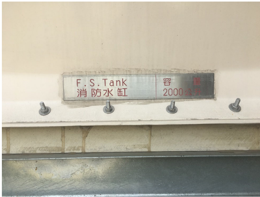
F.S. Tank with 2000L Capacity
