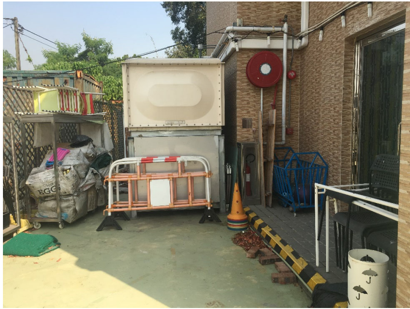
General View of F.S. Tank
