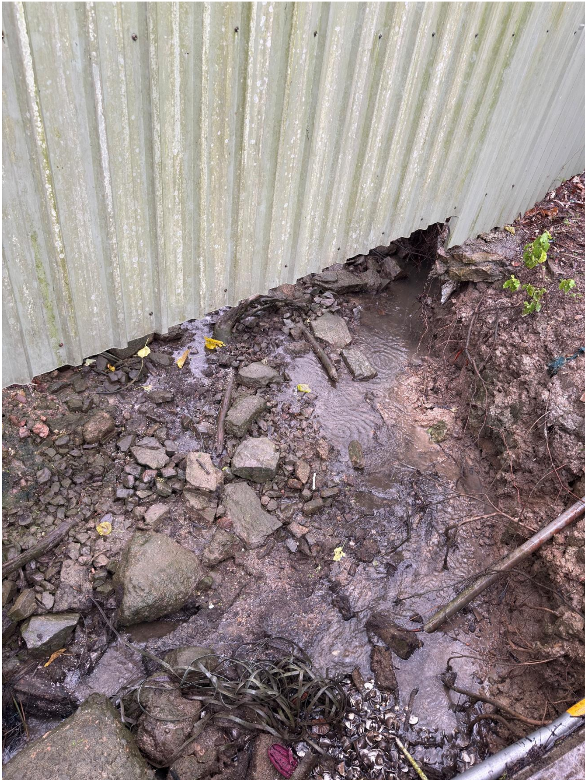
Location of the natural stream on Site (Future location of the Proposed Drainage Pipe M9 to Kam Tin River)
