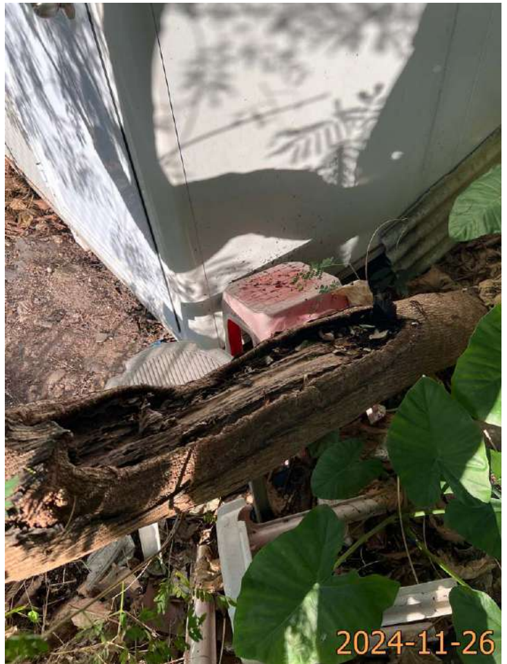
T40 Cavity and decay at trunk
