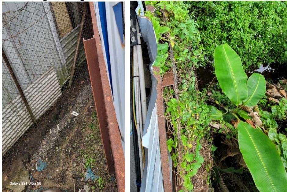
Photos 4 & 5: Natural streams collect the stormwater from the adjacent lots into countryside natural channel.
