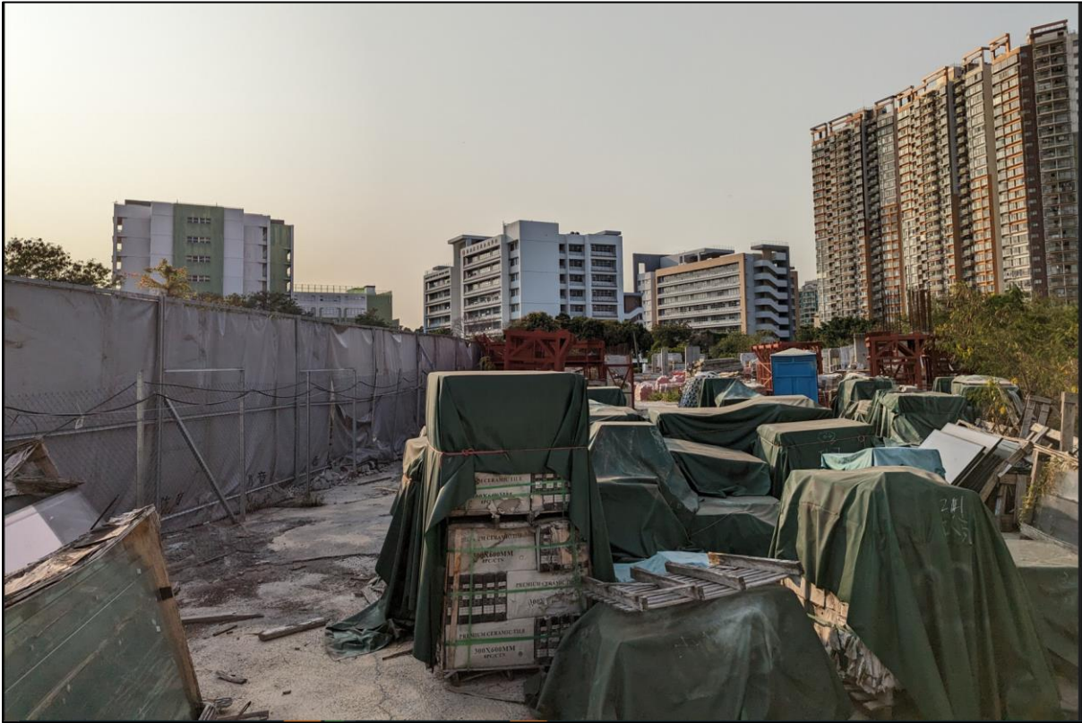
NS 06a: Open Space at the Southwest of the Site – Storage of Construction Material
