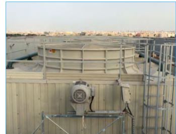
Central Pumping Station Kuwait FWS-500-22-AF x 4
