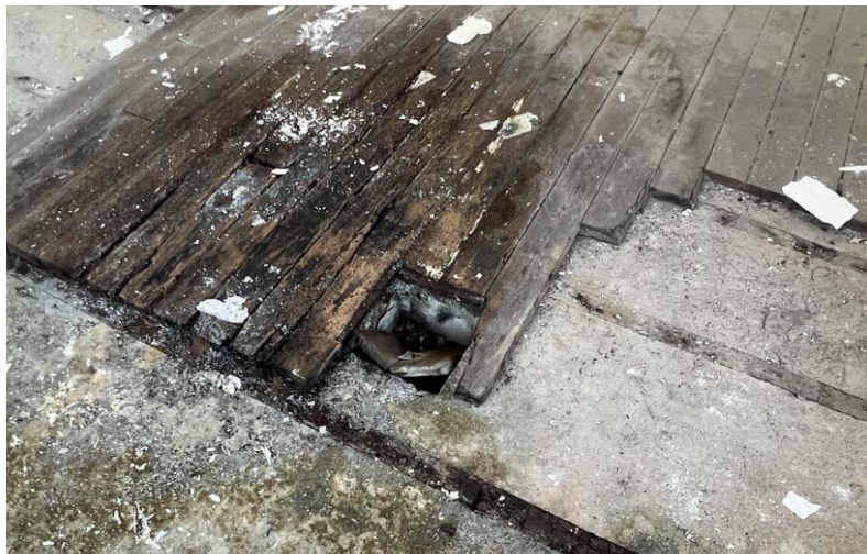
B4.3.37 – A storage space on the floor on the west of the 1/F of Main Building.
