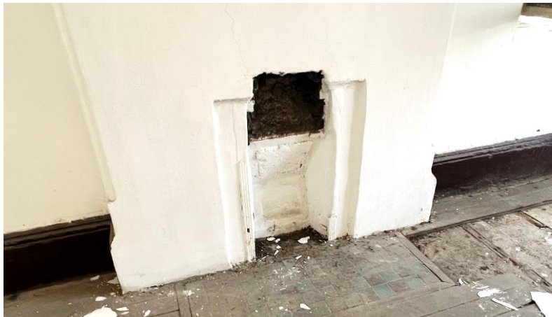
B4.3.34 –The fireplace on the 1/F west side at Main Building of NY.
