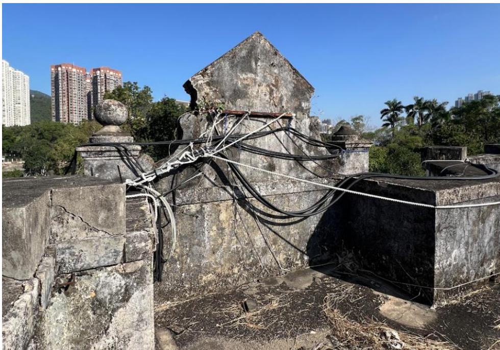
B4.3.4 – Ornate balustrade wall with upstand as observed from the roof level, Main Building.
