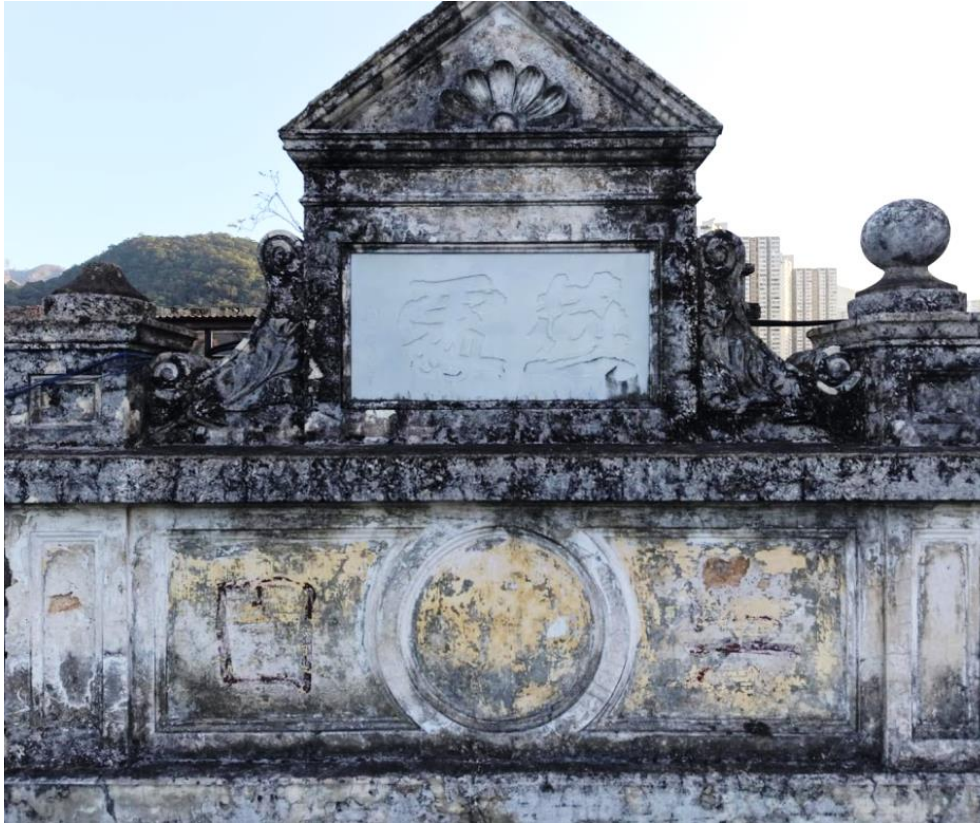
B4.3.3 – Ornate balustrade wall with upstand pediment inscribed with the name and nickname of the residence, Main Building.
