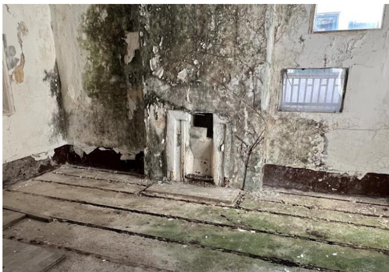
B4.3.35 –The fireplace on the 1/F south side at Main Building of NY.
