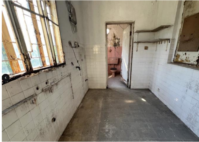
B5.3.3 – The 1/F kitchen with a bathroom at the end as viewed from the interior, Main Building.
