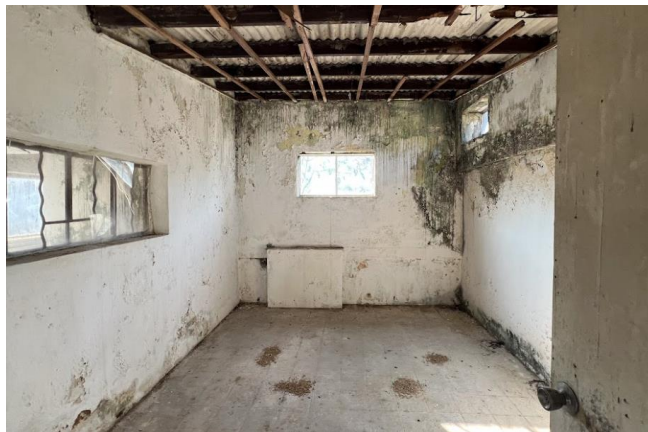
B5.4.4 – This space found on the roof of Main Building is believed to be a bedroom.
