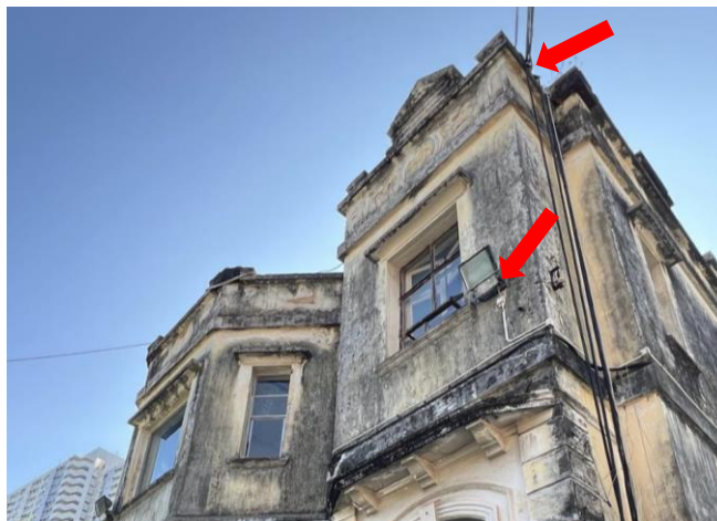
B5.5.1 – Floodlights and electrical cables are found on the facades, Main Building.
