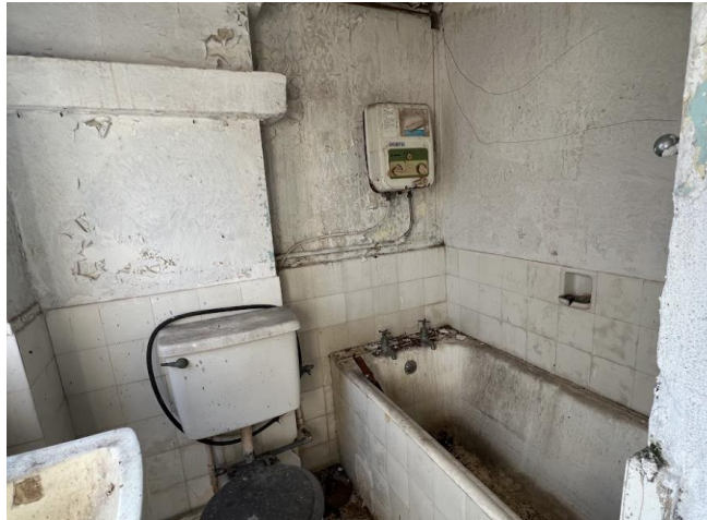
B5.4.4 – The later added bathroom on the roof, Main Building. The toilet is fixed to the roof chimney.
