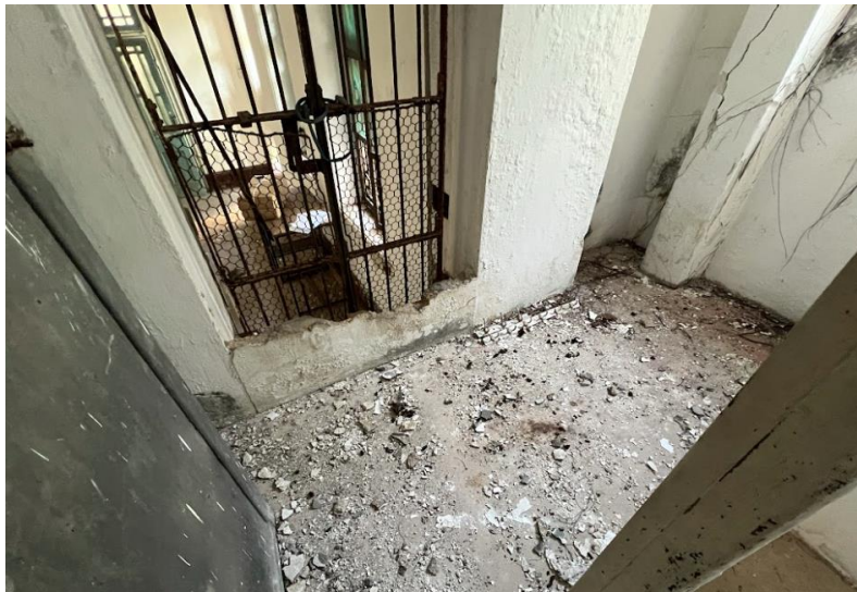
B4.2.13 – View of 1/F store of Sub Building. Original rear entrance with metal fence of NY at the south east of Main Building G/F sitting room is half blocked.
