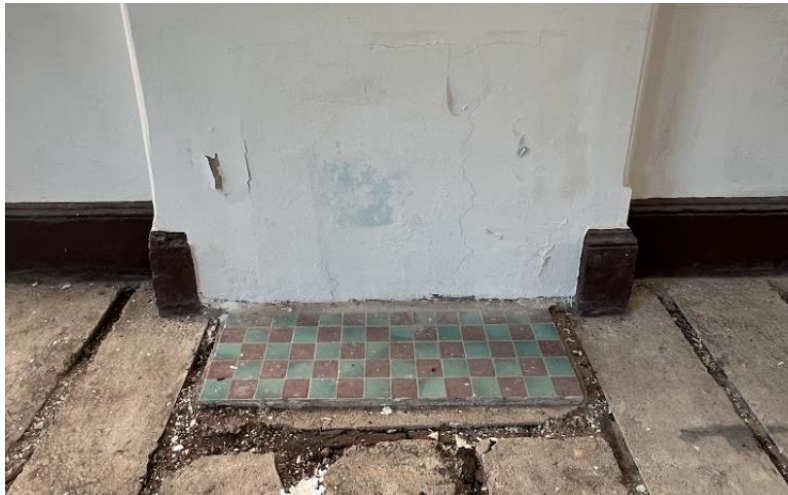
B4.3.33 – The fireplace at the 1/F dining room (east side) at Main Building of NY has been sealed and with the surround removed.
