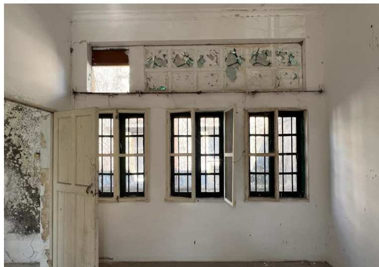
B4.3.15 – Interior view of the 2/F fanlight and windows with metal grilles and mosquito nets, Sub Building.
