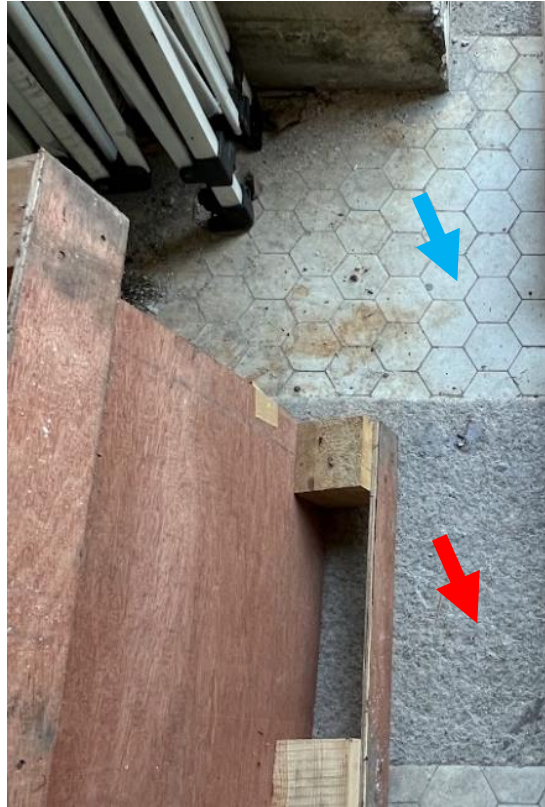
B4.3.17 – Granite (red arrow) and hexagonal tile flooring (blue arrow) at the main entrance porch of Main Building.
