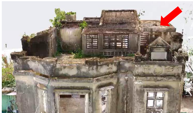
B5.4.1 – The additional structure on the roof, Main Building in 2025. (Source: THE APPLICANT, 2025)
