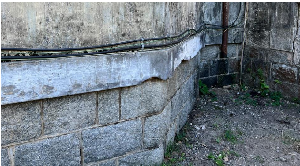
B4.1.3 – Granite to the base of the Main Building which raises the level of its G/F.
