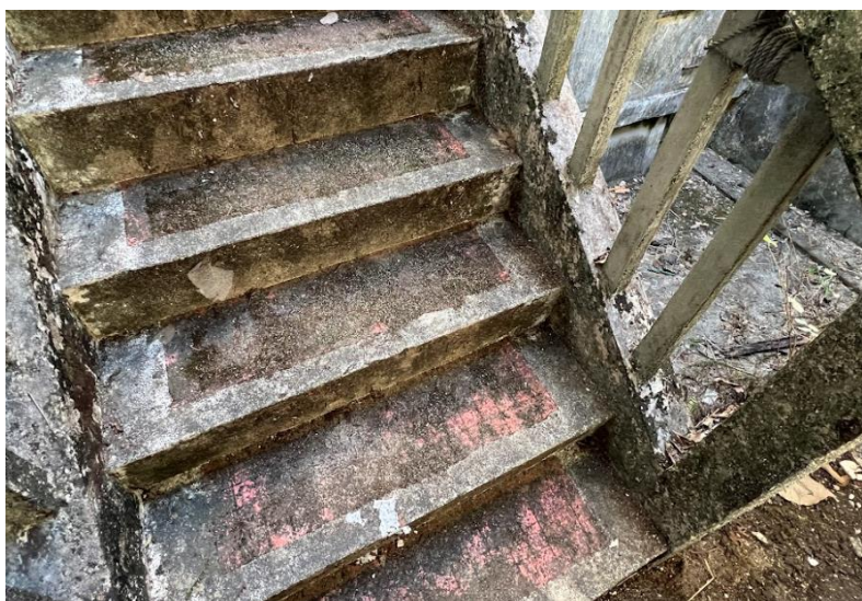
B4.3.29 – Granolithic finish of the external staircase at lightwell, the staircase serves Sub Building only.
