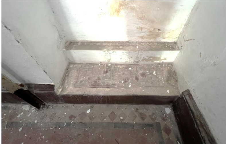
B4.2.12 – The skirting at the staircase landing on the mezzanine level of Main Building was modified for the introduction of a steps that reach the level of the landing between 1/F and 2/f of the staircase at lightwell.
