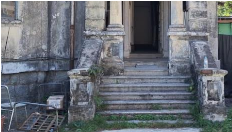
B4.1.2 – Main entrance of Main Building with a small flight of steps.
