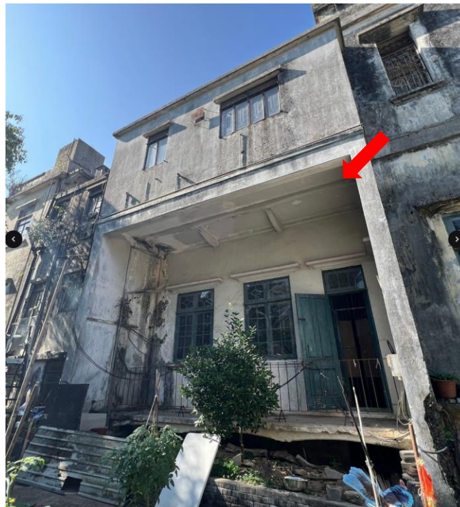
B5.3.2 – The 1/F kitchen and washroom of Main Building as viewed from below. The edge beam with curvilinear profile (indicated by the red arrow) might be the original footprint of the cantilevered bay on the 1/F, providing shelter to the sitting-out area on the G/F.
