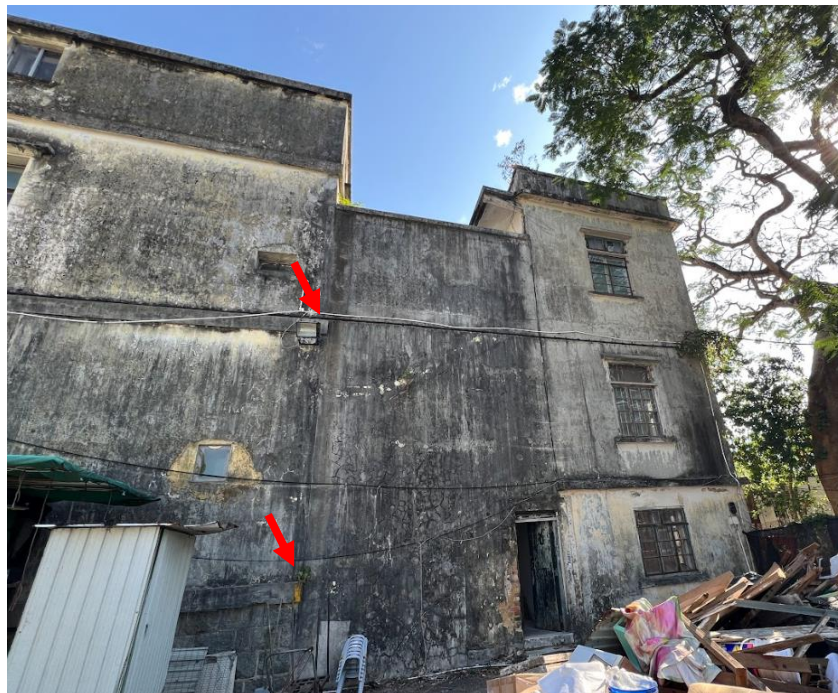
B5.1.1 – String courses of MB wrap around the four sides of MB and terminate abruptly on the side (west) elevation (red arrows) where the later added wall of lightwell is in contact of MB.
