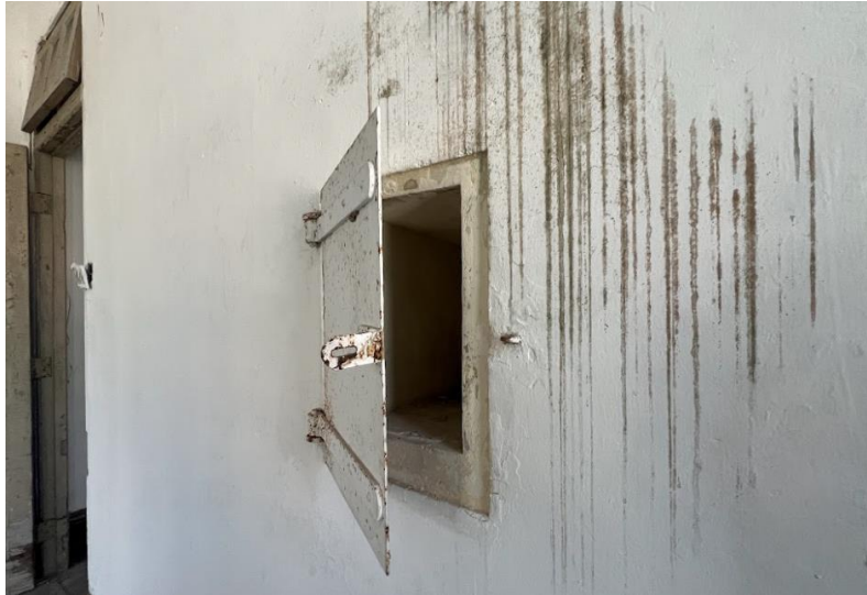
B4.3.36 – A storage space on the wall of the room on the west of the 1/F of Main Building.
