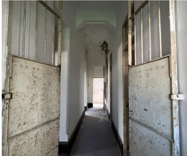
B5.3.4 – The metal gate at staircase landing on Main Building 1/F on which “Private Area. No Entry” are written on both leaves of the gate.
