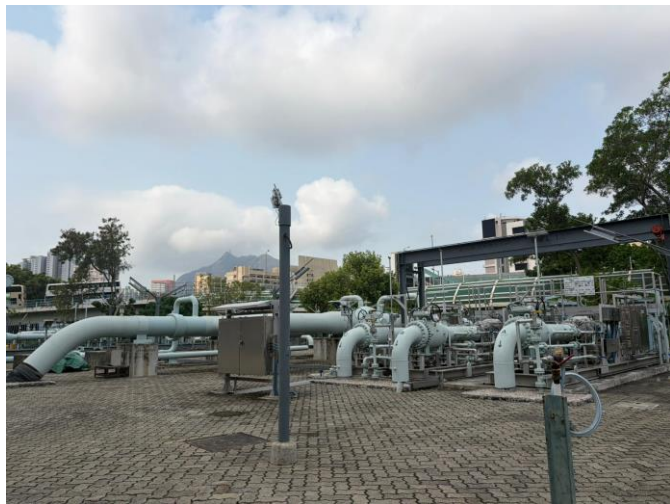
Tuen Mun North Offtake and Pigging Station (P03)
