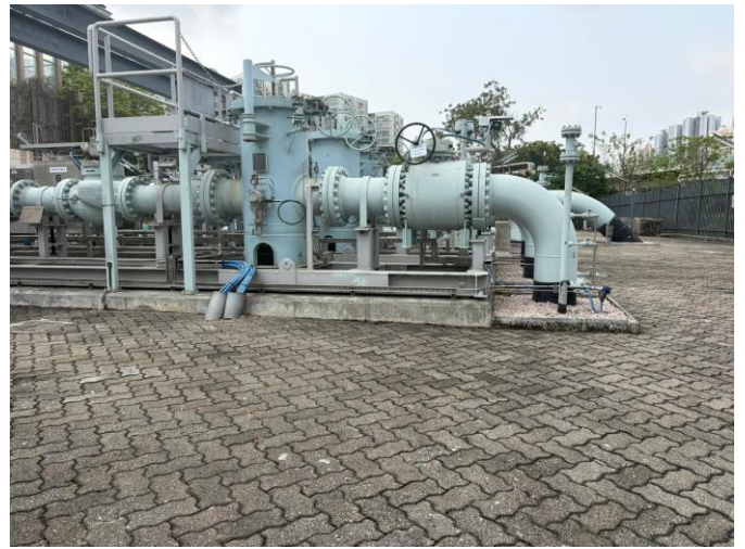
Tuen Mun North Offtake and Pigging Station (P02)
