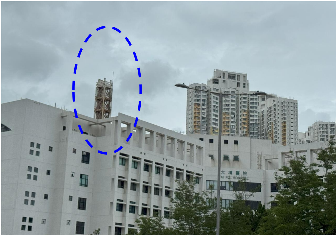
Plate 15: Towngas boilers at Tai Po Hospital (Source ID: TPH02-04)
