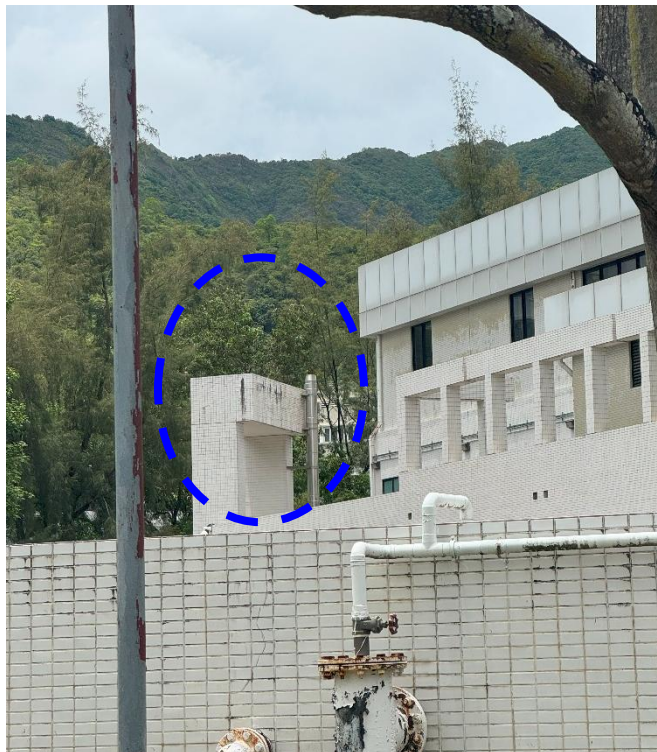
Plate 16: Towngas boiler at Tai Po Hospital (Source ID: TPH01)
