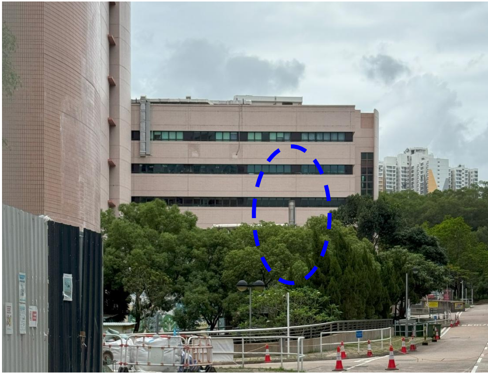
Plate 14: Towngas boiler at Alice Ho Miu Ling Nethersole Hospital (Source ID: NH03)
