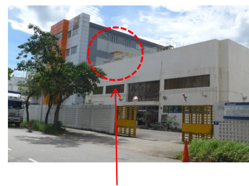
2 cooling towers (rooftop)
