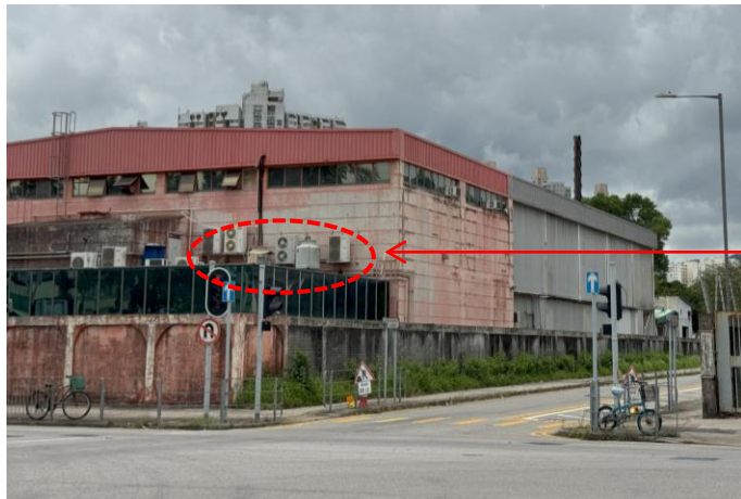
2 cooling towers were observed
