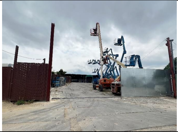
14. Open carpark for crane. No noisy activity or equipment (e.g. forklift) is observed.
