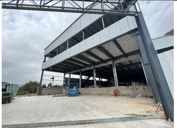
6. Warehouse under construction with no operation is observed. Based on the structure, enclosed warehouse is expected with no potential fixed noise impact.
