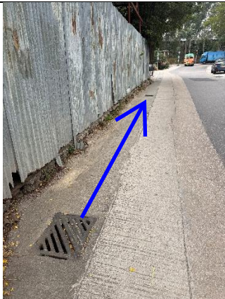
Photo 3 A road gully is located along the southern side of Fung Kat Heung Road and is connected to the natural stream on the eastern side of San Tam Road.
