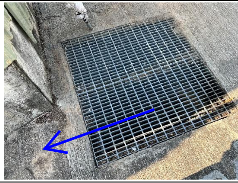
Photo 14 A catchpit is located near the Application Site.
