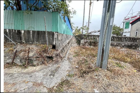
Photo 13 A gully surrounds the warehouse and the logistics company.
