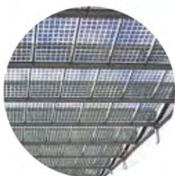
Solar Panels at Block W
