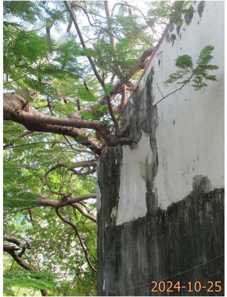
T14 Crown conflict with building
