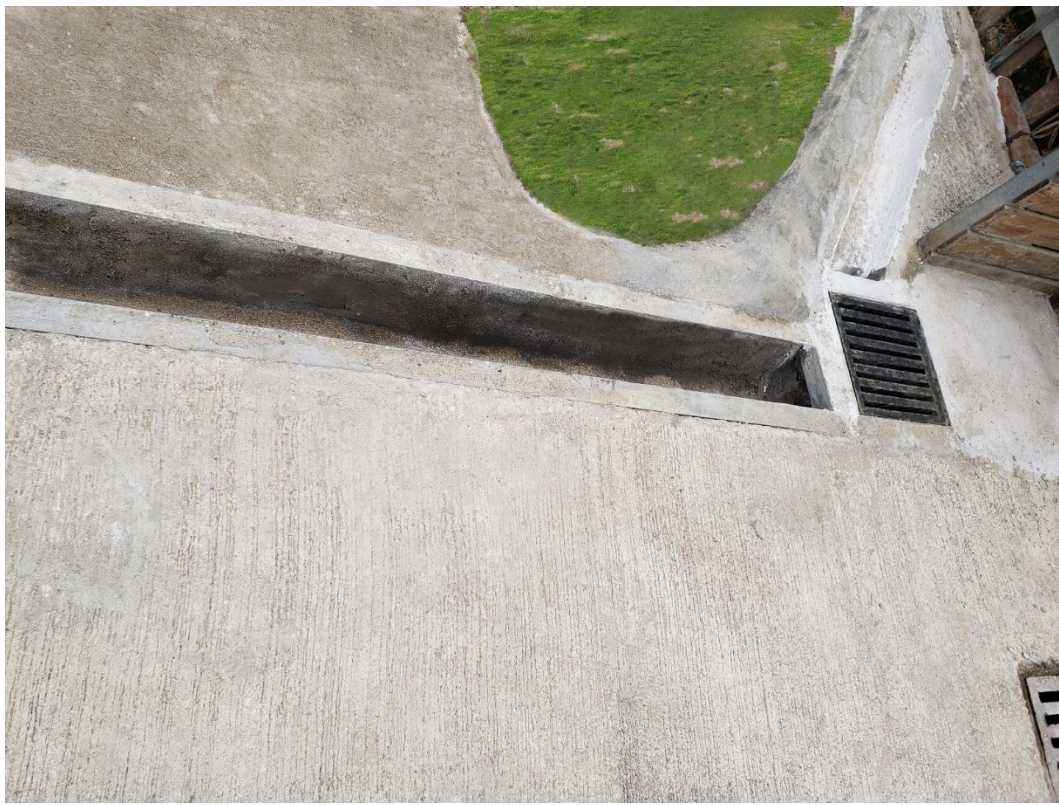
Photo (1) : The terminal catchpit
