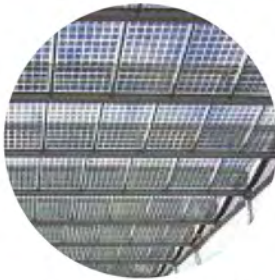
Solar Panels at Block W
