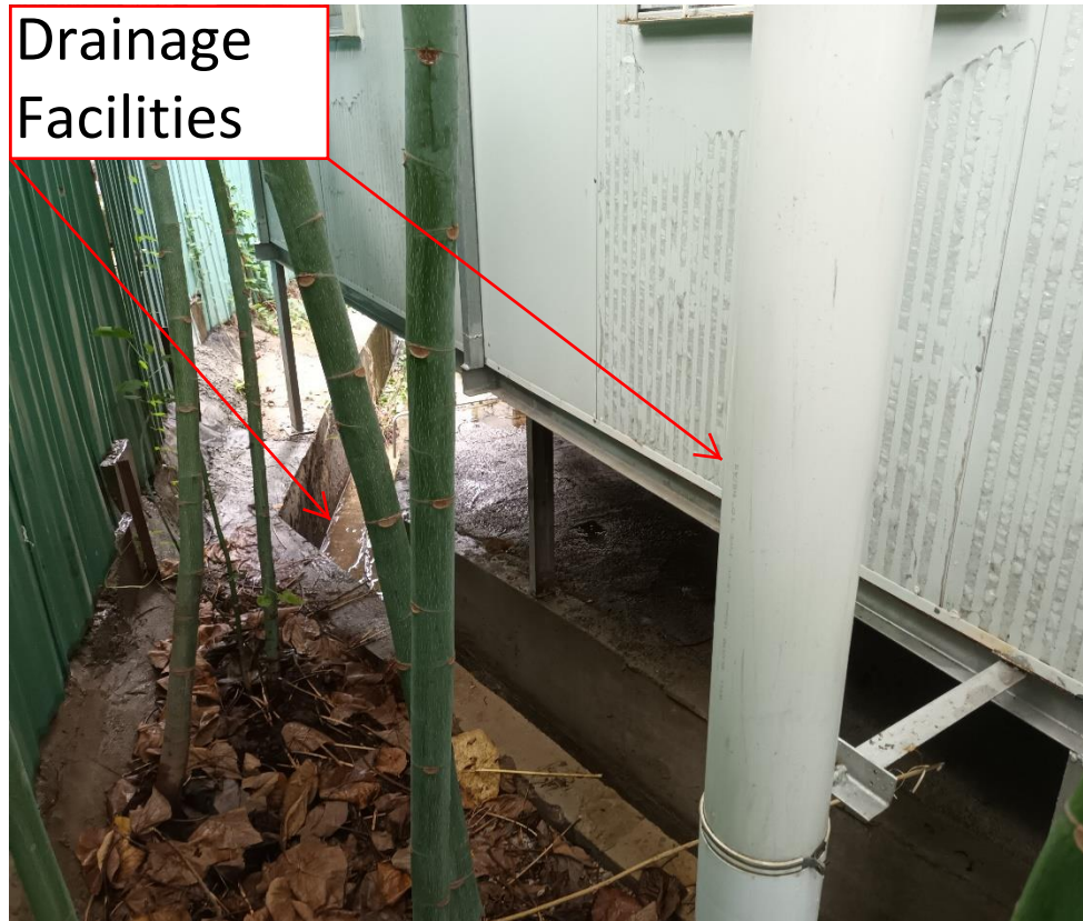
Photo C - Drainage Facilities of Lot 1258
