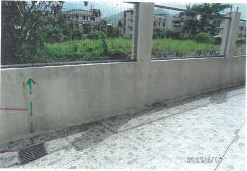
Grating 1. Underground drain
