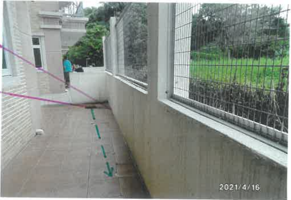
Grating 2. Underground drain
