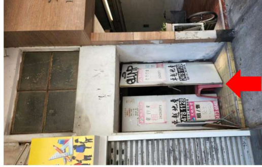
Exclusive Fire Escape Stair Exit
