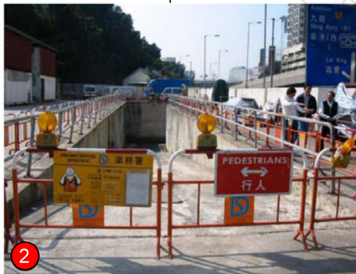
Condition of ramp covers
